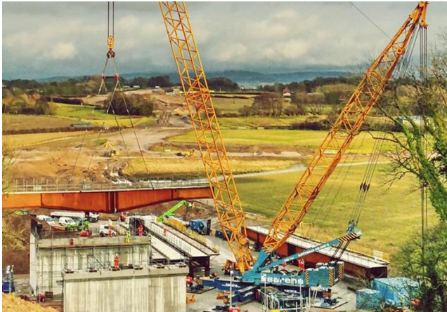
An 850-tonne crane was used to lift the steel beams into place over a 6-day period.
