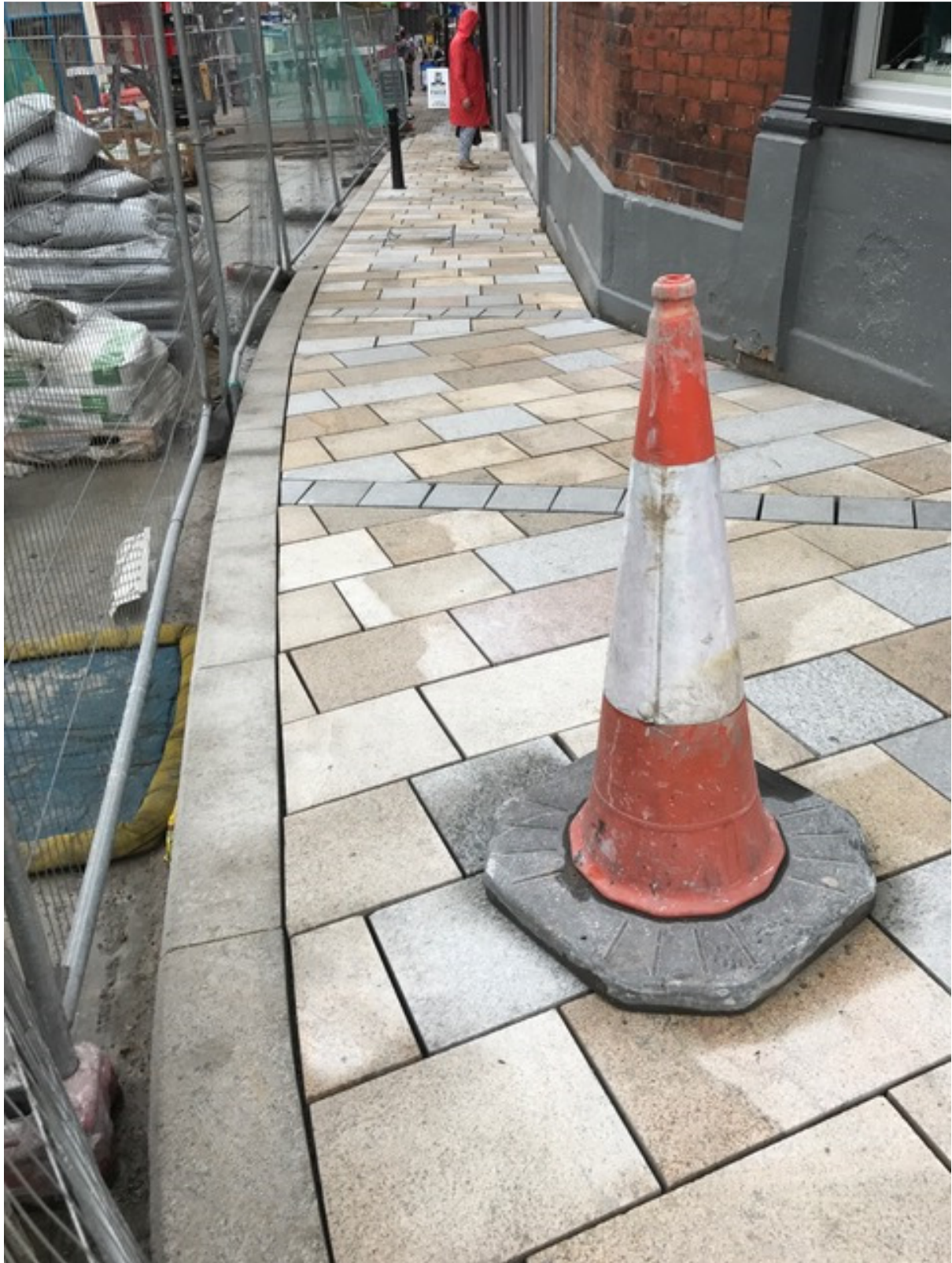
Photo Number 2 shows the new granite paving at the south east footway adjacent to Duke Street.
