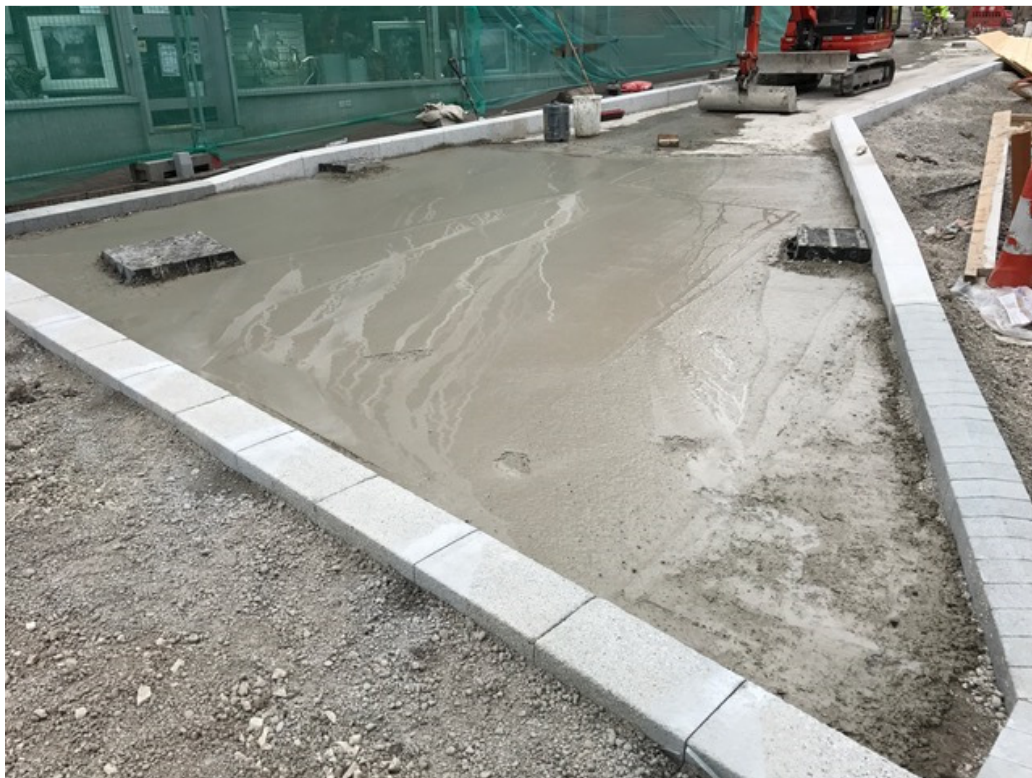
Photo number 3 shows the installation of the concrete foundation at Duke Street for the new carriageway.
