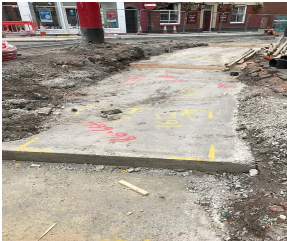
Photo number 4 shows the installation of the concrete foundation for the new granite bench.
