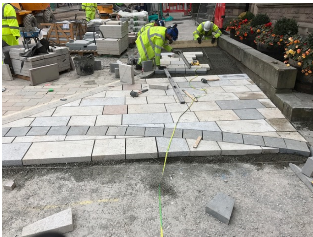
Photo number 5 shows the installation of new granite paving for Swan Bank footway.
