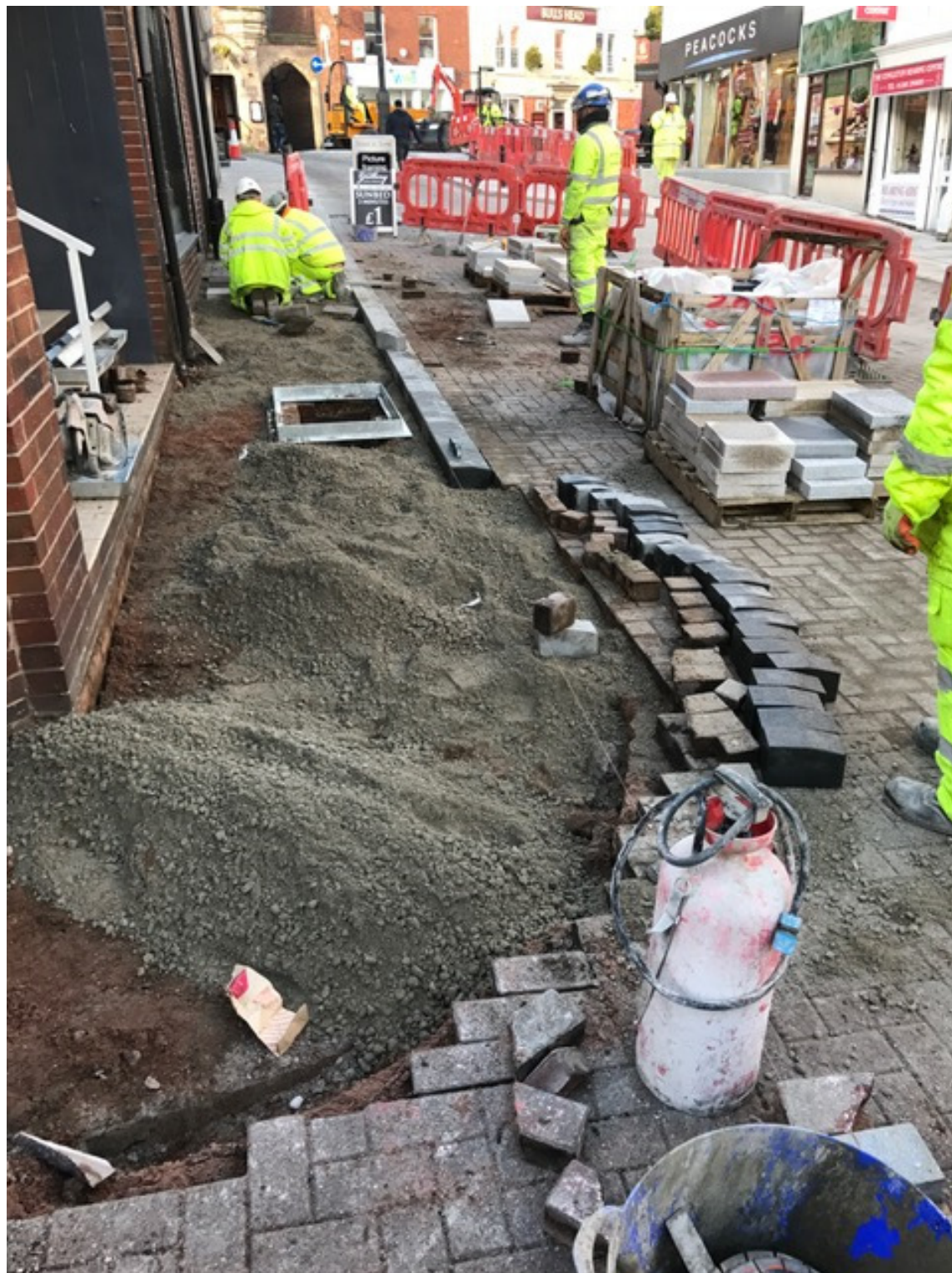
Photo number 3 shows the excavation of the south footway between Swan Bank and Little Street.
