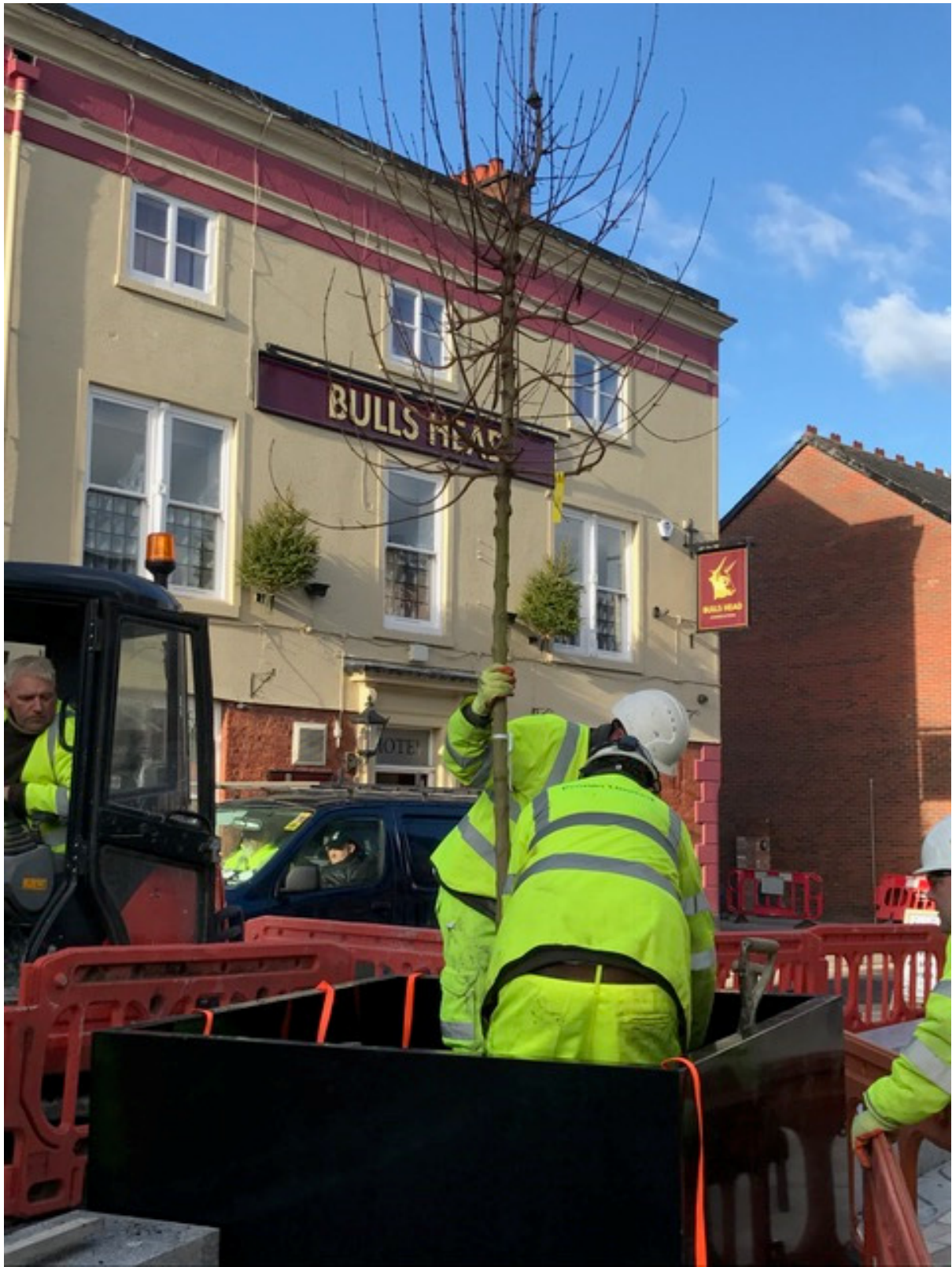
Photo number 4 shows the installation of the trees in the new planters at Swan Bank.
