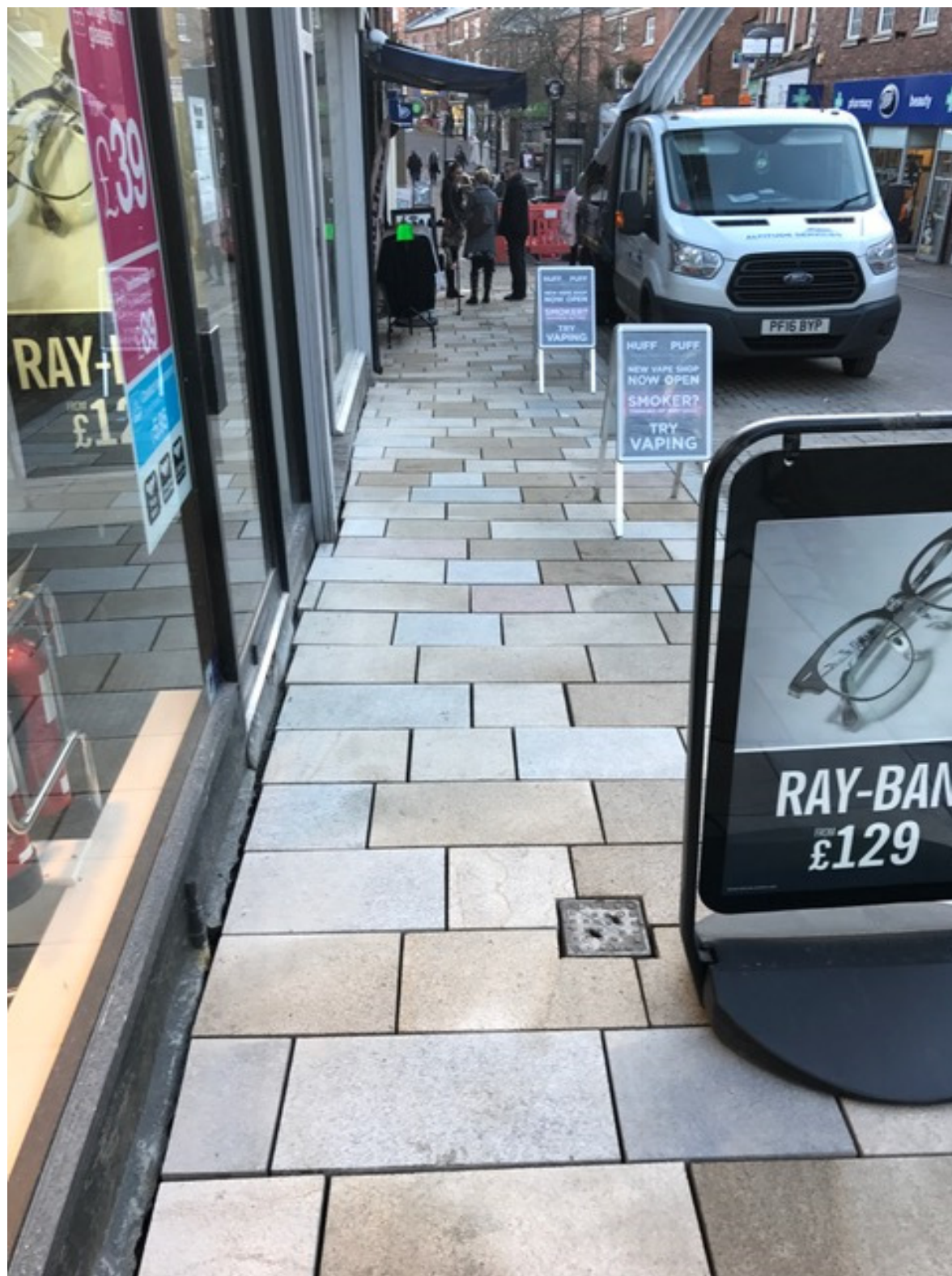
Photo number 2 shows the installation of the new granite block paving on the north footway between Swan Bank and Victoria Street (looking east towards Victoria Street).
