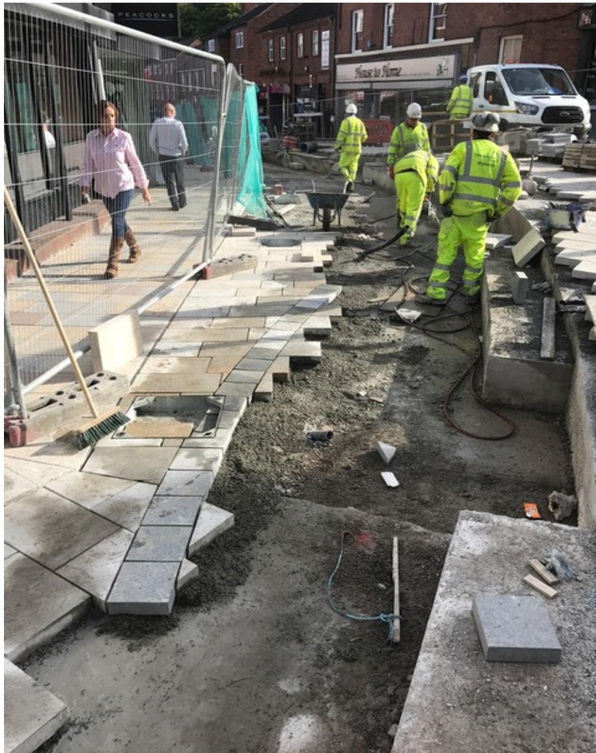
Photo Number 2 shows the new granite paving at the north east footway adjacent to Duke Street.
