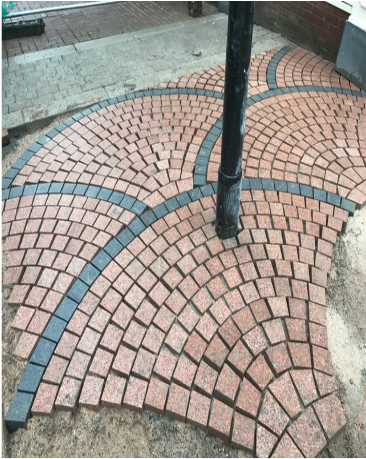
Photo number 2 shows the newly installed granite paved 'fan' pattern at Victoria Street.
