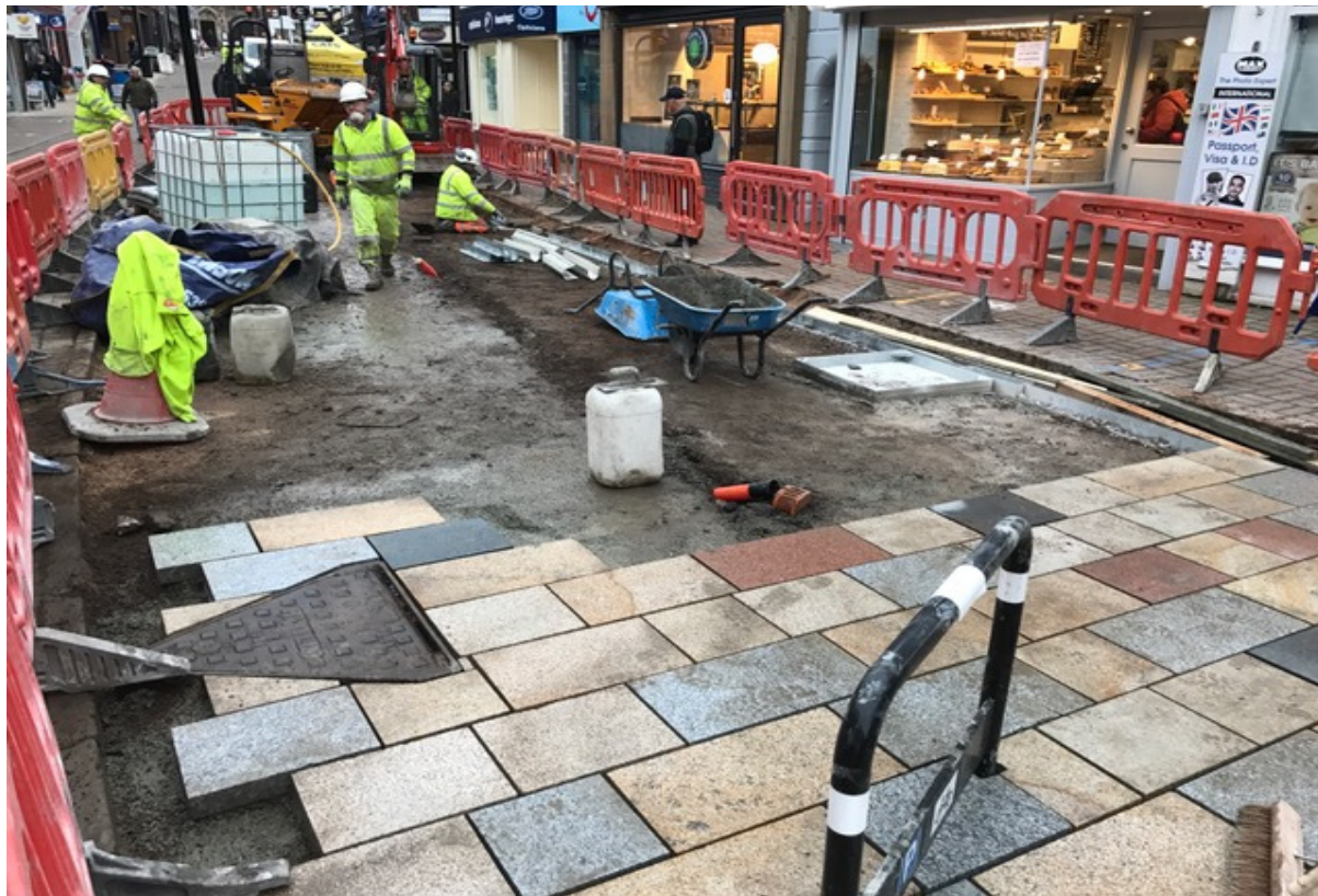
Photo number 3 shows the excavation works and the installation of the new slot drain.
