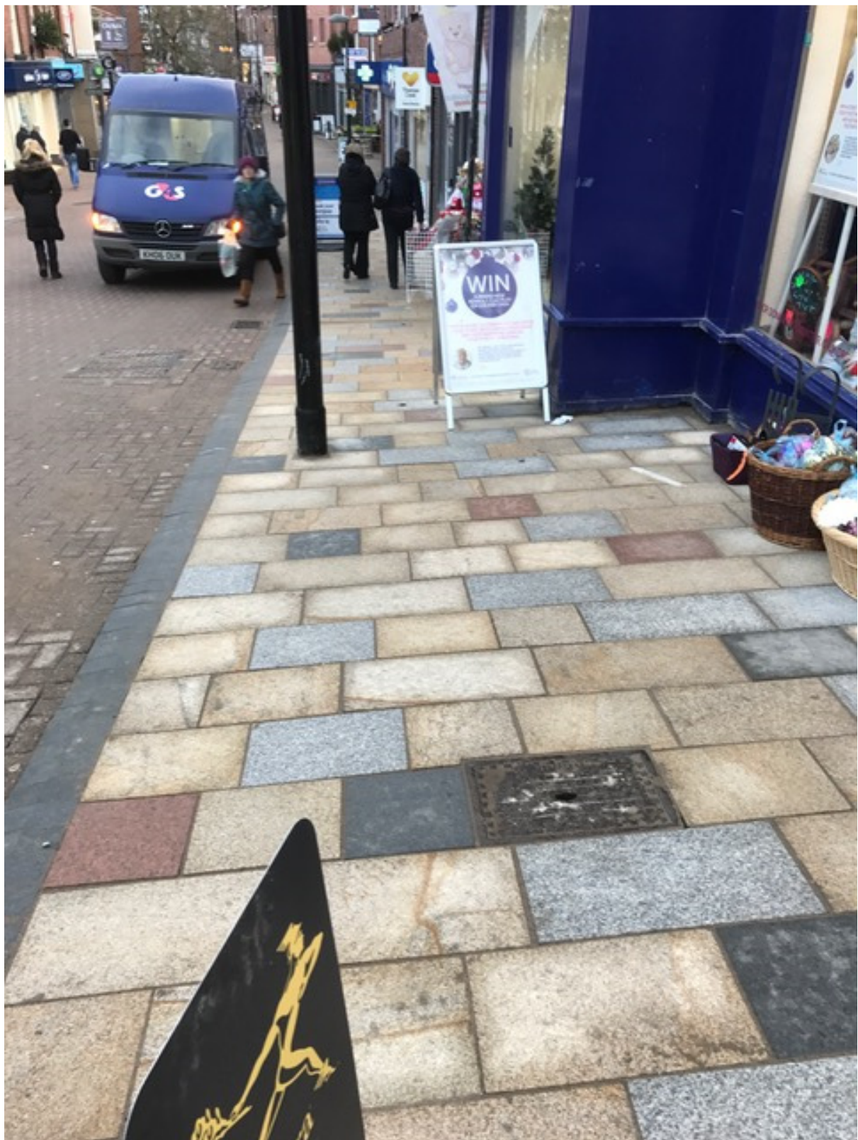
Photo number 2 shows the freshly grouted granite paving on the south footway
