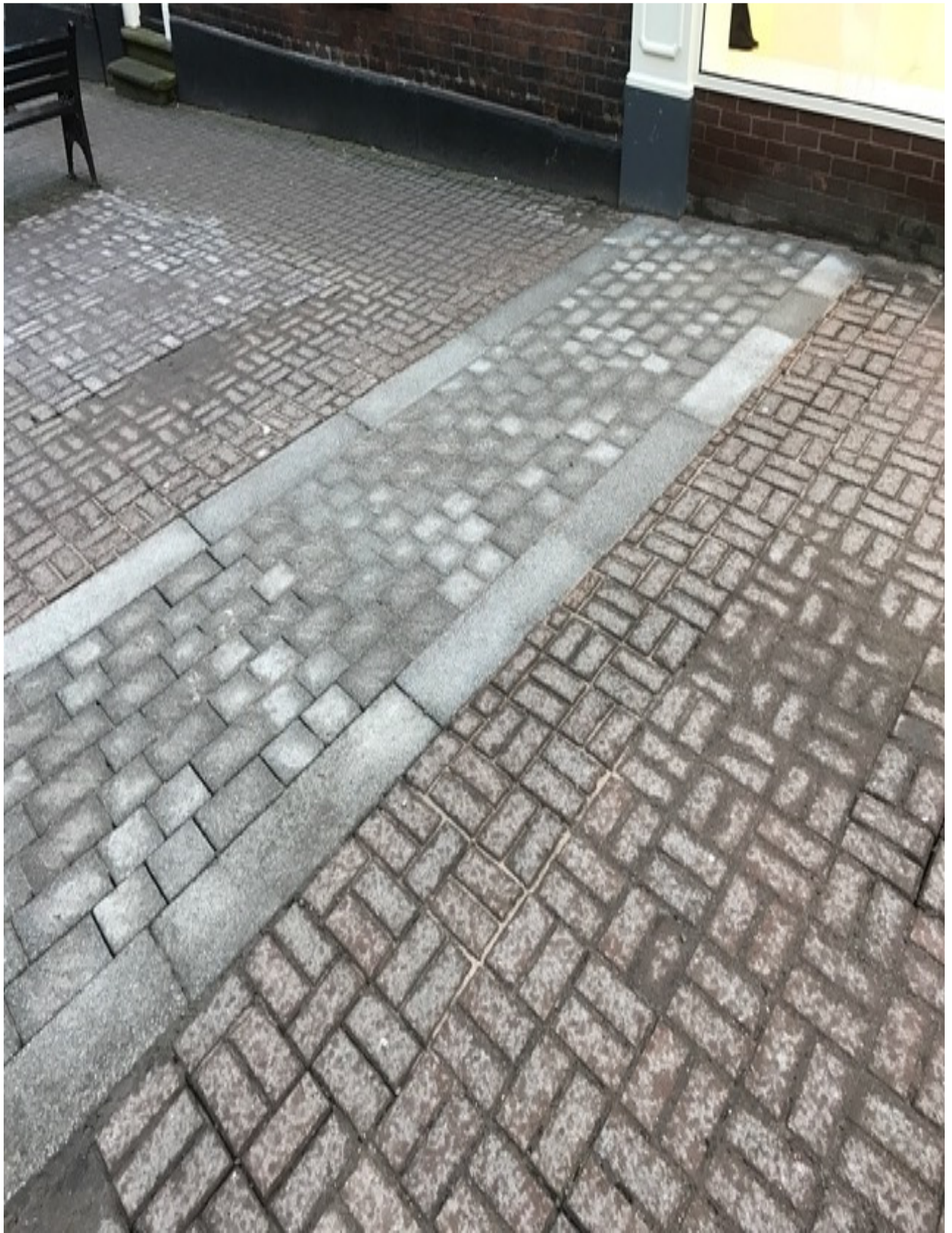
Photo number 3 shows the installation of the transition detail at Victoria Street.
