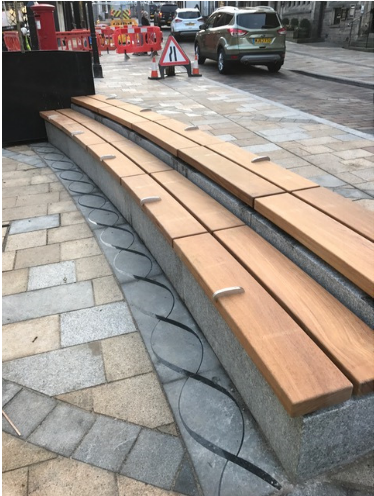
Photo number 4 shows the installation of the new timber seating on the granite bench..
