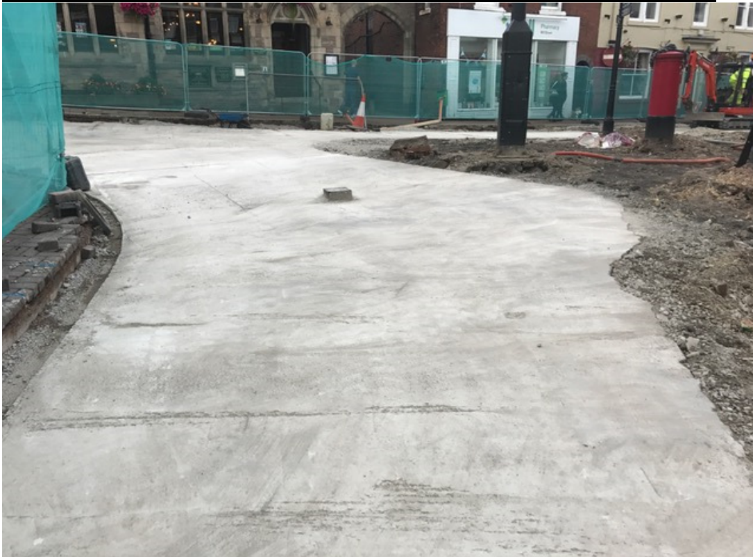
Photo Number 2 shows the new concrete base for the carriageway at Duke Street
