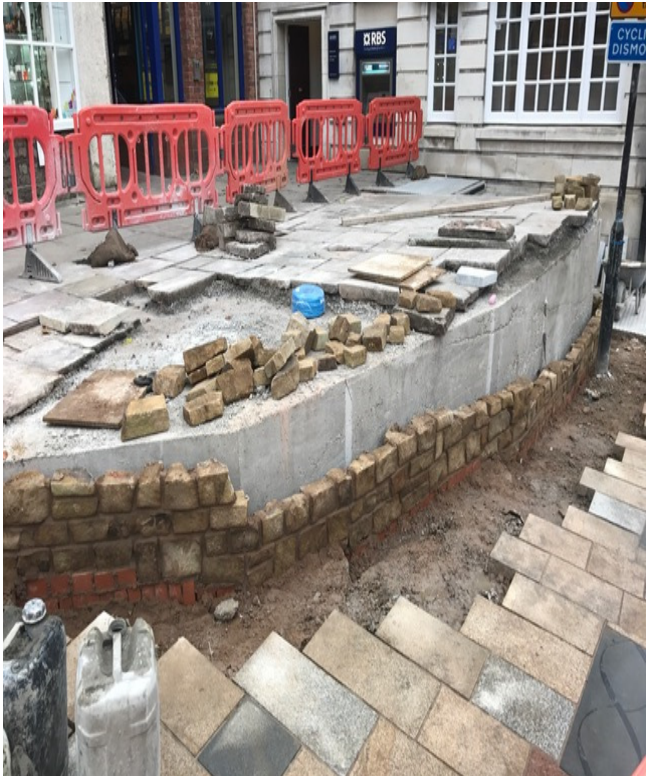
Photo number 3 shows the construction of the new wall at the south west footway (RBS Bank).
