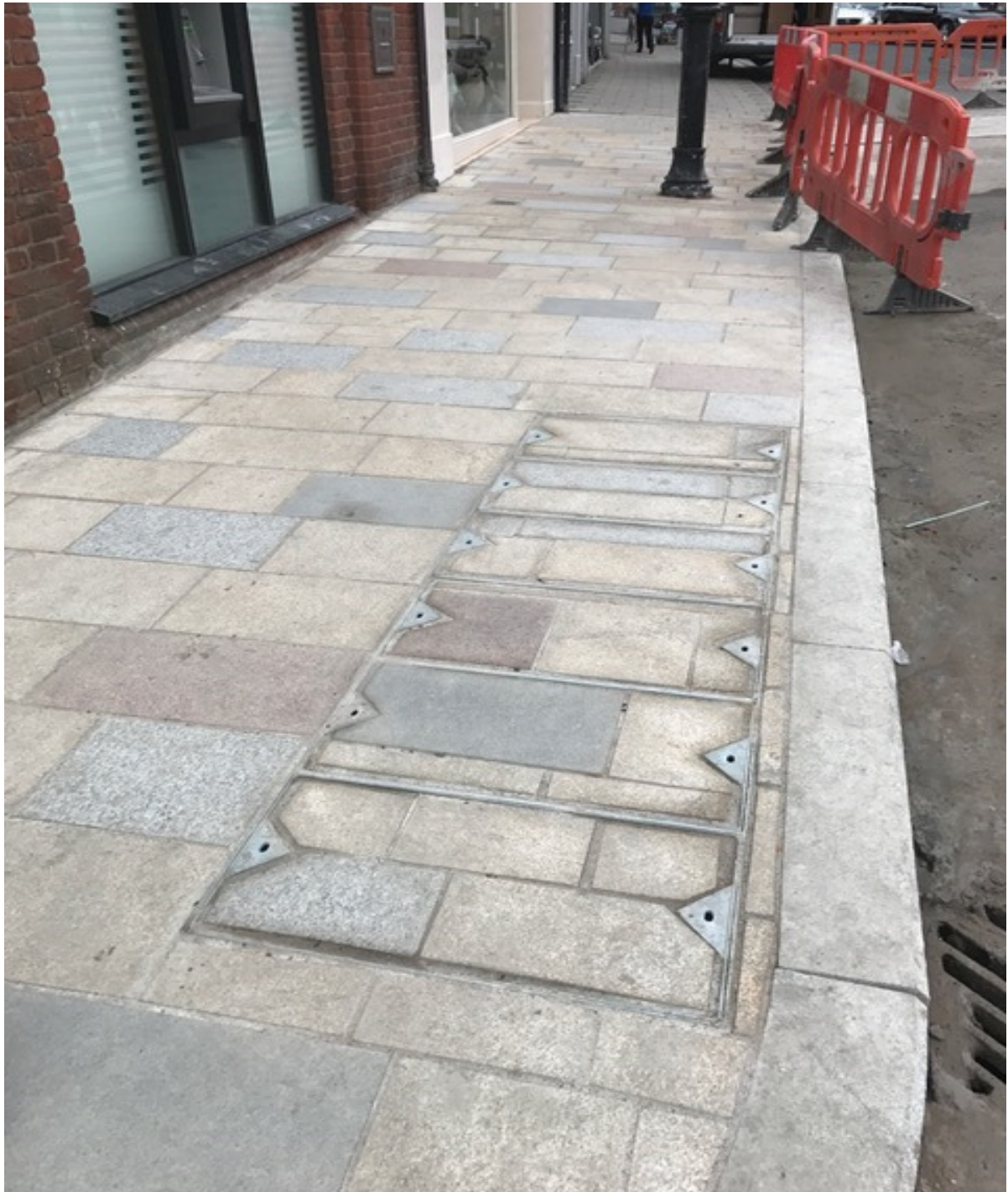
Photo Number 2 shows the new kerbline and granite paving at the north east footway (Barclays Bank).
