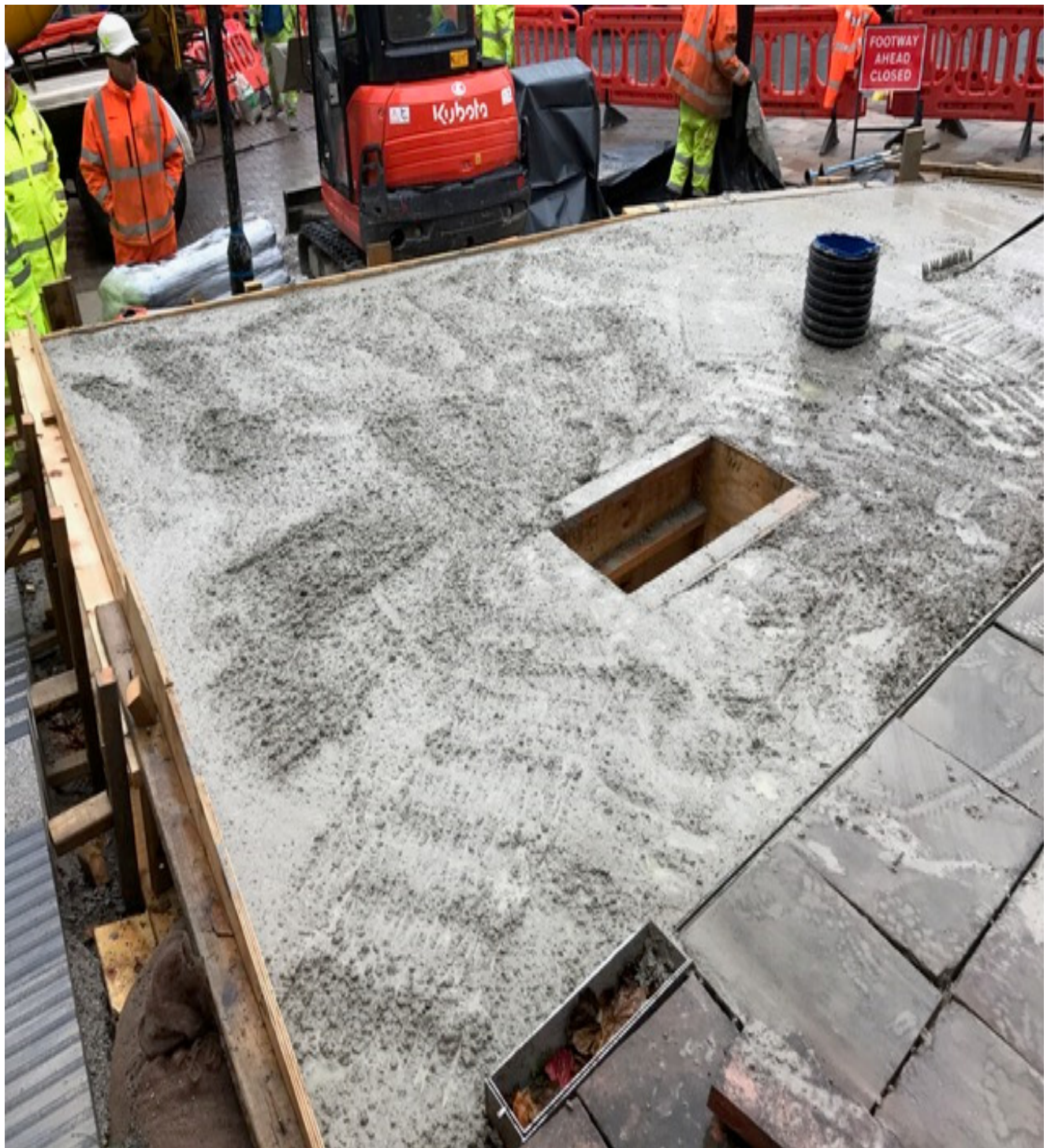
Photo Number 2 shows the concrete pour for the Woolies Wall, including the socket for the Christmas Tree.
