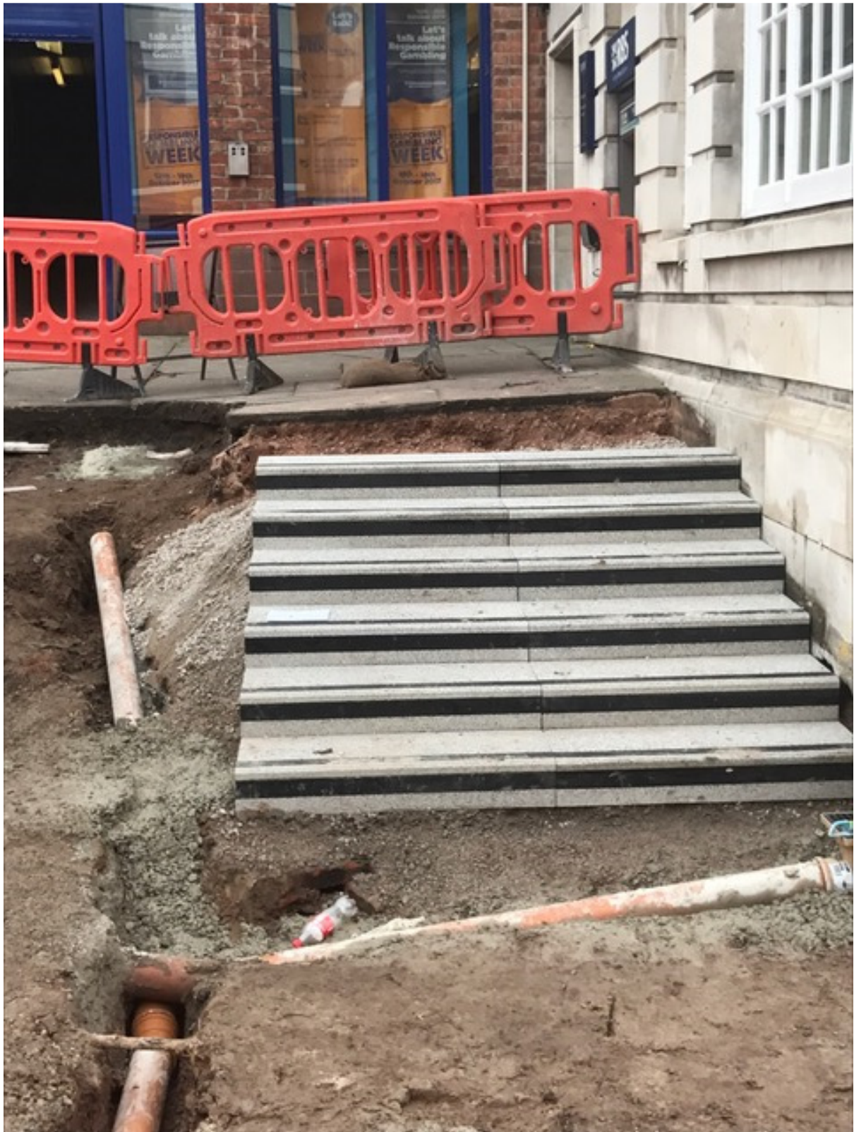
Photo number 3 shows the installation of the new granite steps leading up to the RBS Bank.
